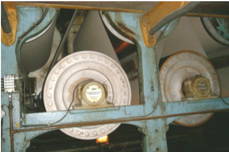
The drying section at Romiley Board Mill.
